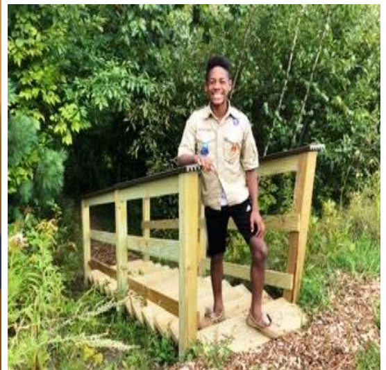
Walter Fegel designing and building new stairs to the Pond Learning Center.
